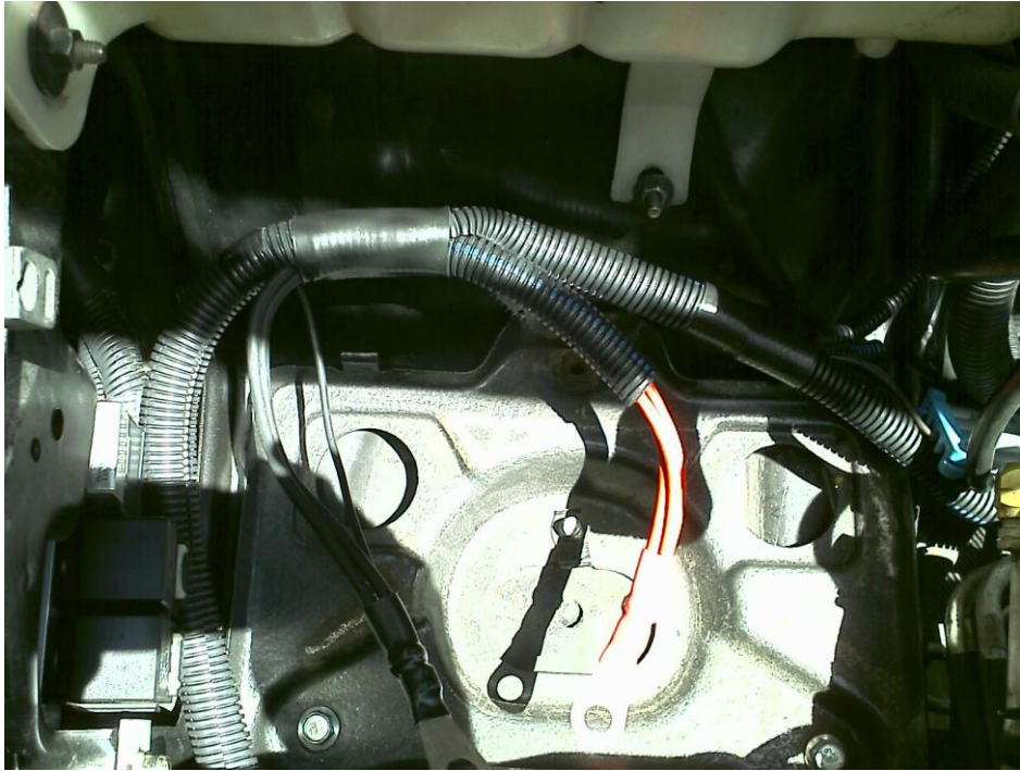
Wire routing over to the battery and fans.
