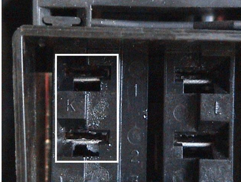
40 amp fuse holder terminals.
